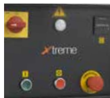
Low voltage (24V) control panel with star-delta system
